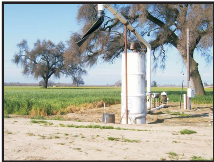
Irrigation well & discharge to pipeline
