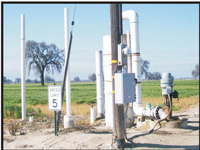
Canal lift pump
