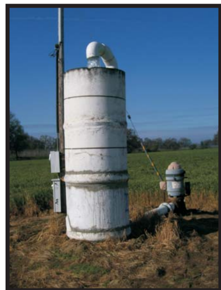
Irrigation pump & well
