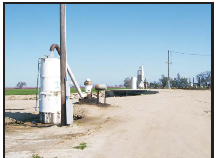
Irrigation well & lift pump in background
